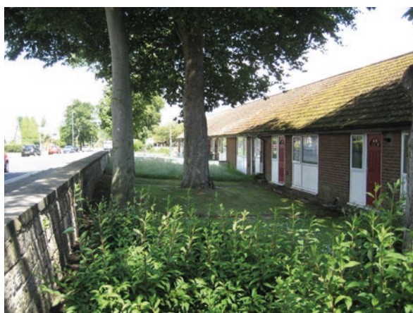
Poor relationship: background chestnut tree at just 4m from the front of the dwelling (guideline distance 10m). Trees are overbearing and cutting out light even though they are on the N side.
