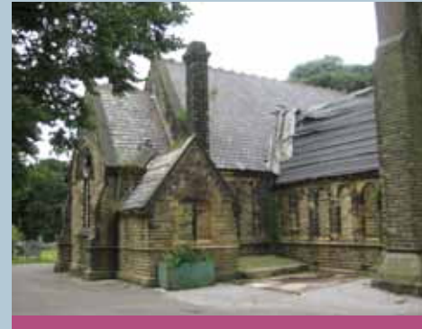
Chapel within the grounds of Pudsey cemetery showing severe signs of dilapidation and also with missing roof slates
