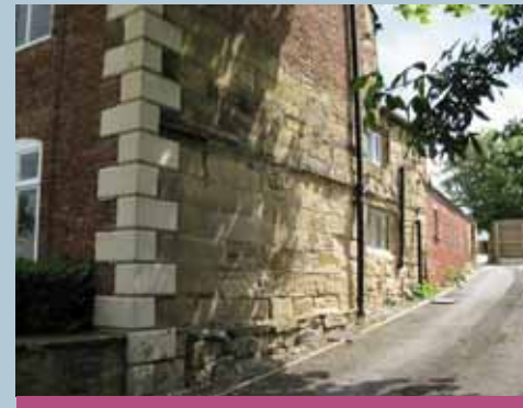
Long Acre incorporates the remains of a 17th century building in its western side elevation
