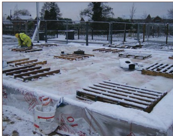
Figure A4.84 Taped joints are difficult to construct in adverse weather. Also difficult to inspect if covered with snow (courtesy Smith Grant)
