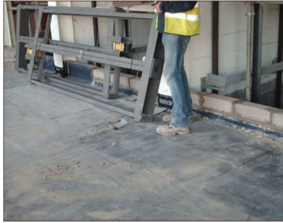
Figure A4.50 Large/heavy/sharp objects being moved over unprotected gas membrane (courtesy Card Geotechnics Limited)
