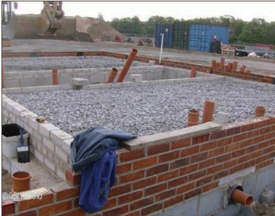
Figure A4.85 Clean single sized stones with no fines acting as venting media, however no ventilation gaps in internal sleeper walls (courtesy Smith Grant)
