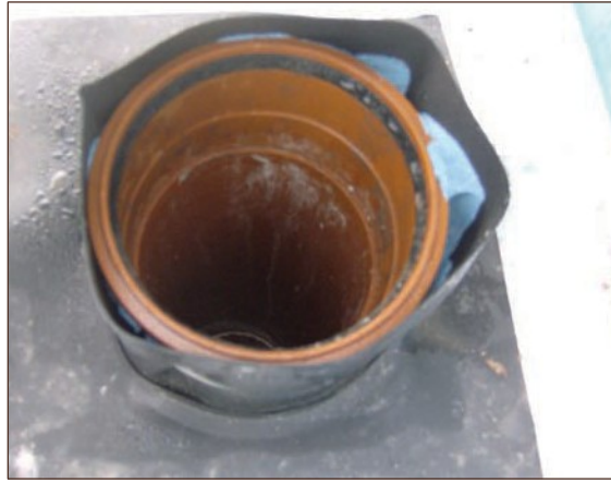
Figure A4.74 Gap between OD of service pipe and ID of top hat too large: cannot be compressed enough to form seal, even with the application of additional tape (courtesy Smith Grant)
