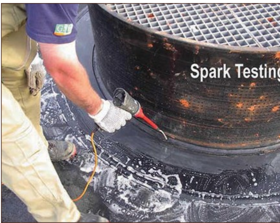
Figure A4.45 Spark testing (courtesy GSE Environmental)
