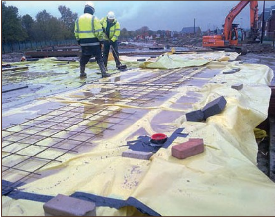
Figure A4.67 Traffic over mesh resulted in several punctures, in addition most joints were found to be poorly constructed. Taped joints are difficult to construct in adverse weather (courtesy Smith Grant)
