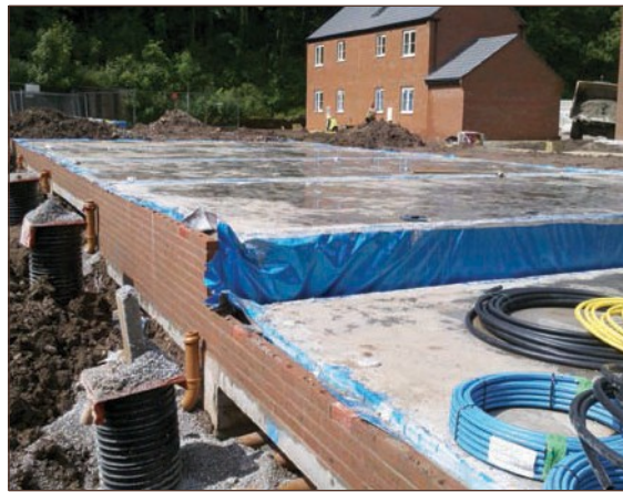
Figure A4.82 Gas membrane used to bridge cavity wall instead of DPC, leaving it exposed to damage by follow-on trades (courtesy Smith Grant)
