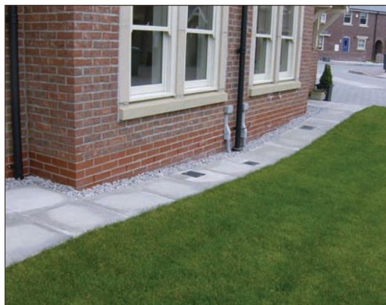
Figure A4.36 Raised air bricks are preferable due to the reduced potential for blockage but the vent trench specified is provided with clean single sized stone (courtesy Smith Grant)
