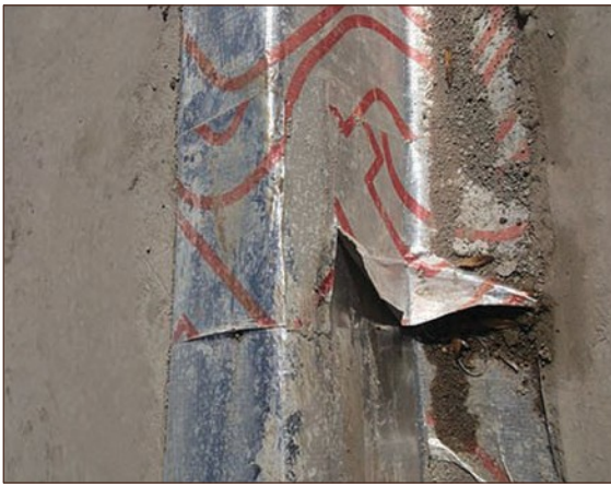
Figure A4.55 Gas membrane at stepped junction of slab to integral garage, appears to be susceptible to tearing when screed is poured. Screed may also weigh down on gas membrane if fitted too tight (courtesy NHBC)
