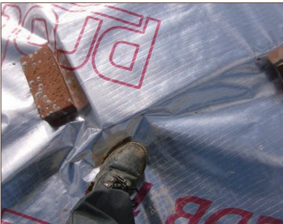
Figure A4.71 No corner detailing leading to stress point on gas membrane (courtesy Smith Grant)
