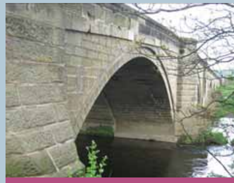
The existing Pool Bridge, built in 1754, with alterations in 1801 and 1812. The rebuilding of the bridge would have reflected increased traffic in the area.
