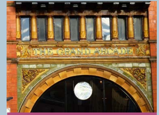
Colourful, locally made Burmantofts faience and art nouveau detailed terracotta (below left) at The Grand Arcade
