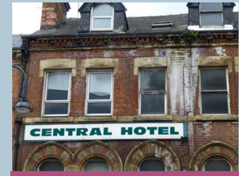
Unaddressed maintenance issues get progressive more harmful and expensive to resolve
