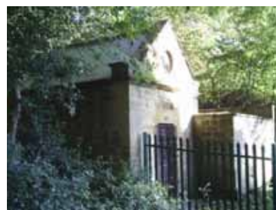
Gipton Spa needs repairs.
