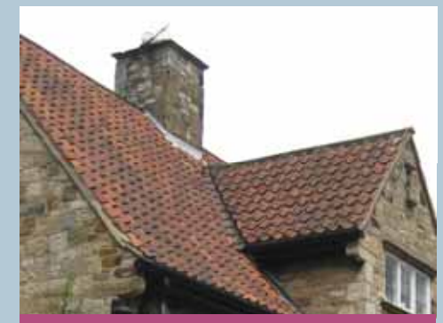
The use of pan-tile and slate is important to retaining a traditional appearance of the roofscape.
