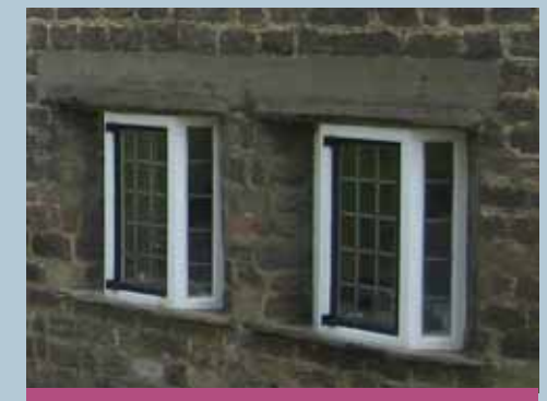
This splayed window detail was commonly employed by William Alban Jones in Linton during the early 20th century.
