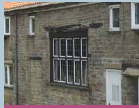
By not disguising rural elements of buildings, such as this former cart opening, the rural character is maintained.
