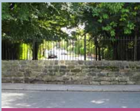
Field boundary wall incorporated into the later West Park development, Spen Road
