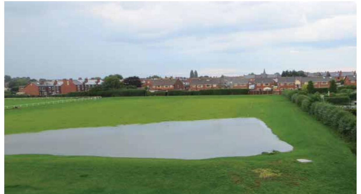
BARLEY HILL RECREATION GROUND FLOOD WATER STORAGE: AN EARTH EMBANKMENT REDUCING FLOOD RISK TO 20 HOMES AND PROPERTIES. FRM WORKED CLOSELY WITH PARKS AND COUNTRYSIDE TO ENSURE THE WORKS WOULD NOT IMPACT ON THE NEARBY FOOTBALL PITCHES. ADDITIONAL FENCING WAS ALSO INSTALLED TO MAINTAIN PRIVACY TO NEARBY HOMES.
