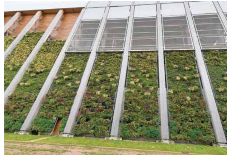
GREEN WALL, VEOLIA RECYCLING AND ENERGY RECOVERY FACILITY
