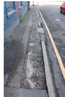
Poor quality surfacing
