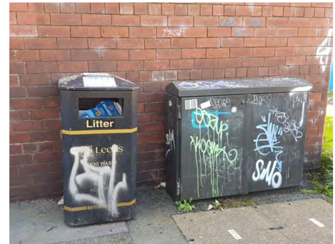
Bin and telecoms cabinet in a poor condition, Regent Street character area
