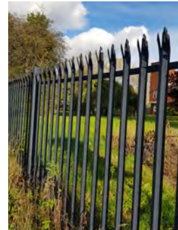
Typical intrusive security railings
