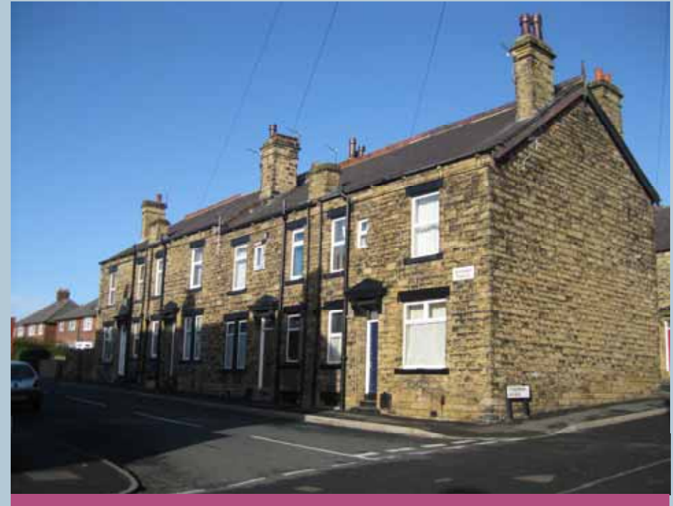
Fine detailing such as stone lintels and ornamental door pediments should be sympathetically repaired and maintained if the character is going to be preserved, such as here.
